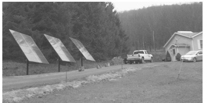
Solar panels installed at DCEC member Frank Eppich’s home
