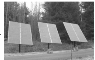
Solar panels installed at DCEC member Frank Eppich’s home
